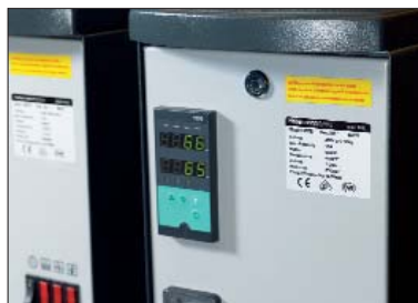
Professional type plate on a heating unit.
