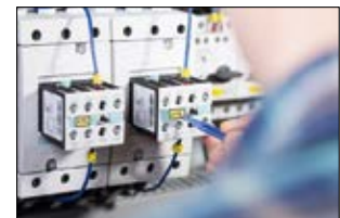
Safety and clarity in control cabinets with HELASIGN labels.
