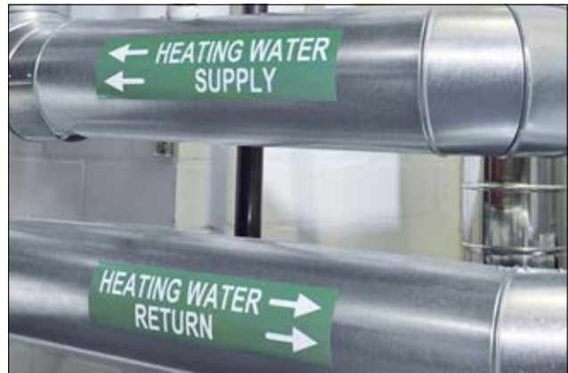
Large and highly visible pipe marking.
